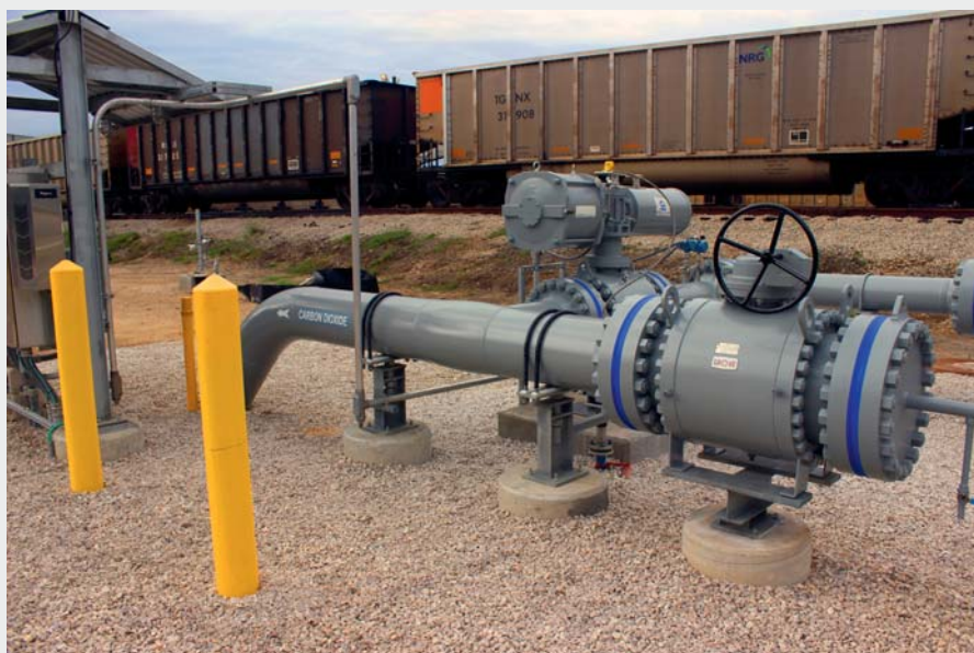
Petra-Nova CO 2 supercritical pipeline. Copyright NRG Energy.
