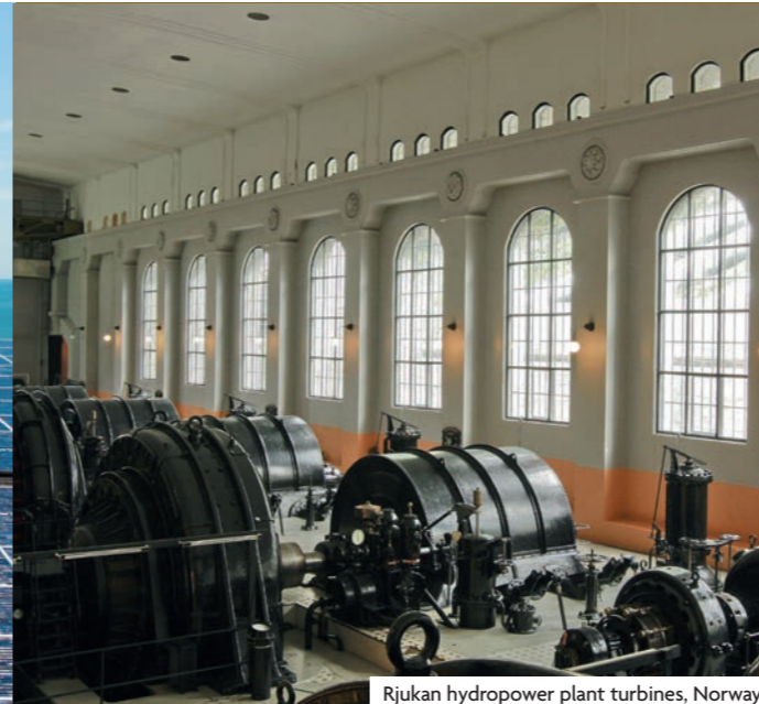
Rjukan hydropower plant turbines, Norway
