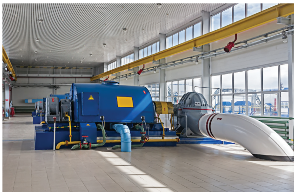
Gas compression stations are a major source of methane emissions in the oil and gas sector
