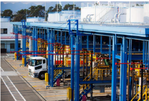
Figure 3. Refined products or chemicals transfer from bulk storage to road tankers requires gas detection.
