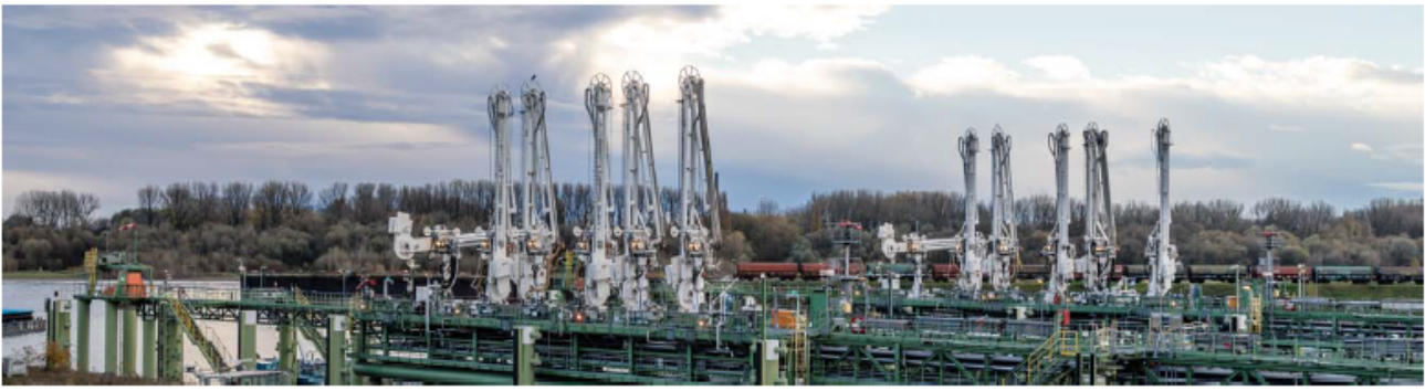
Figure 1. Flammable or toxic product transfer from land-based storage to and from barges or tankers is common on inland waterways in Central Europe.
