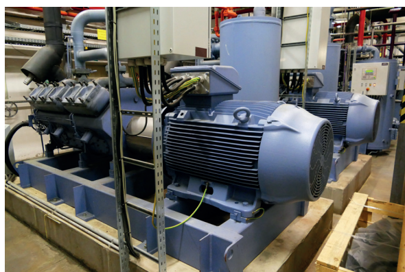
Ammonia refrigeration compressor
