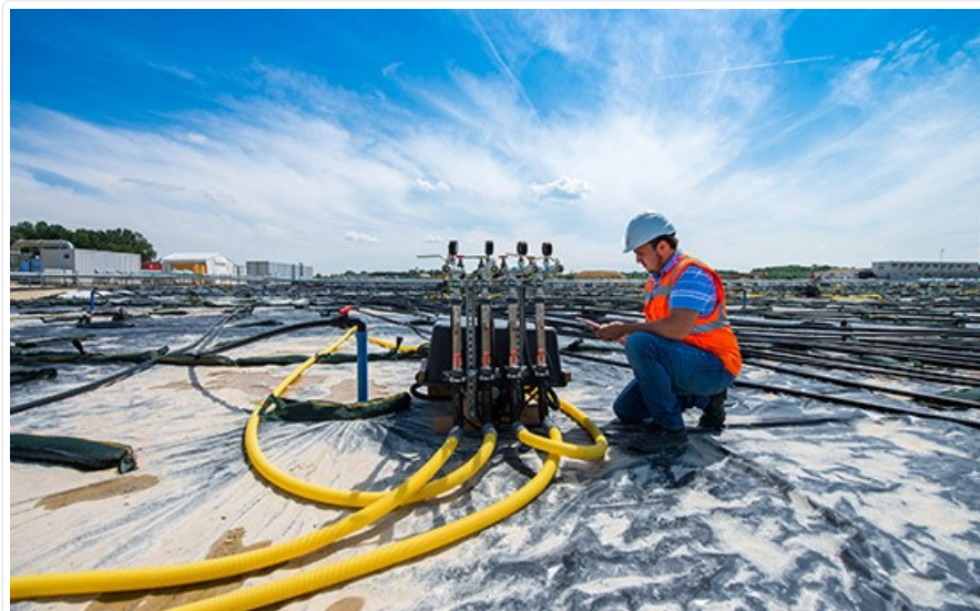
IN-Campus Environmental remediation of legacy refinery at Ingolstadt - air sparging unit (copyright AUDI AG).
