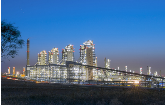
Image courtesy of Air Products and Chemicals Inc. Four gasification reactors at Lu'an, China
