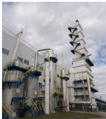
Air Separation Unit
