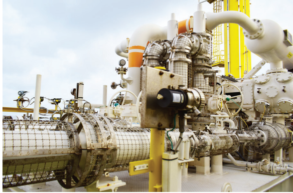
Fixed flammable gas detection
