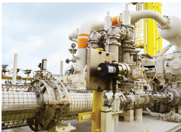
Fixed flammable gas detection system
