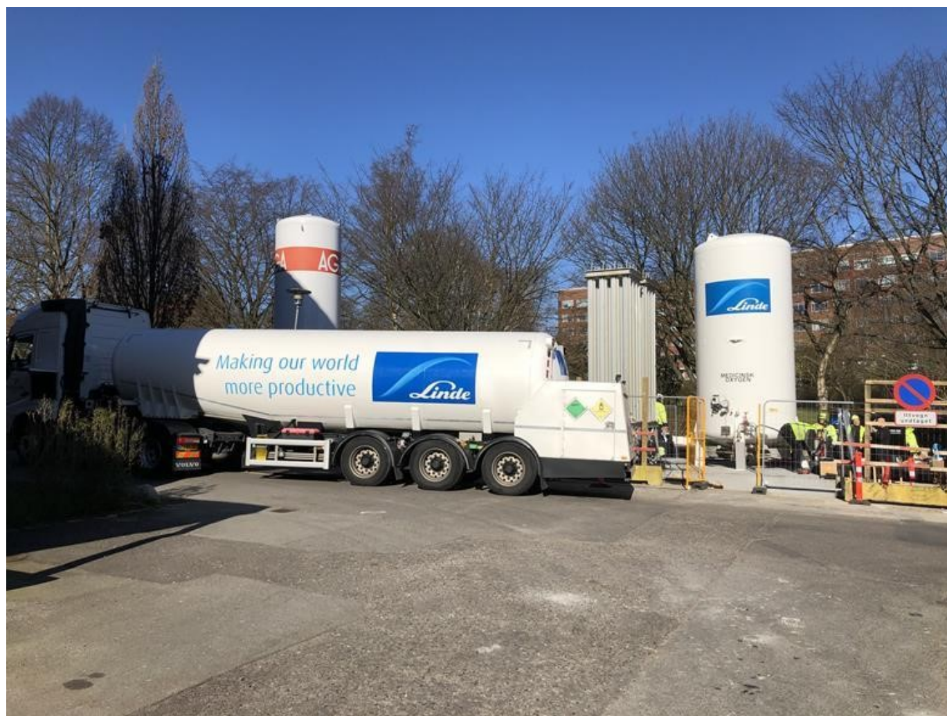
Source: Linde Bisbebjerg hospital installation
