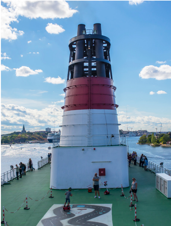
Marine CEMS systems are installed in the ship's funnel
