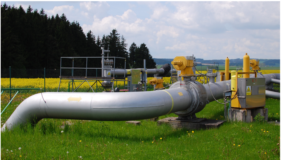
Natural gas distribution pipeline
