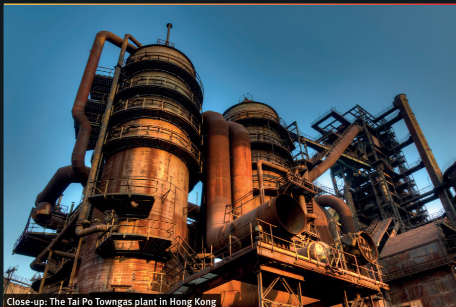
Close-up: The Tai Po Towngas plant in Hong Kong
