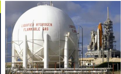
Liquid hydrogen storage at Cape Canaveral
