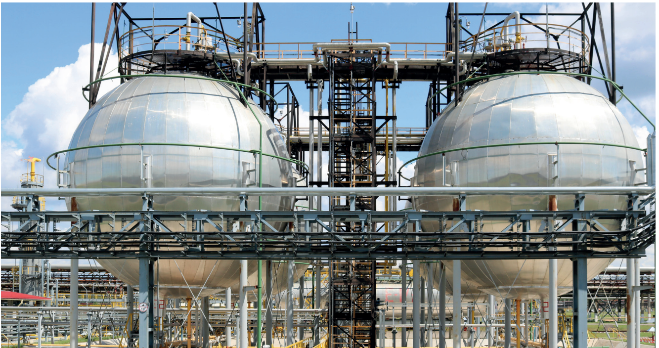
Above: Ammonia storage spheres
