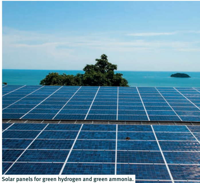
Solar panels for green hydrogen and green ammonia.
