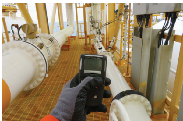
Hand-held portable gas leak detection
