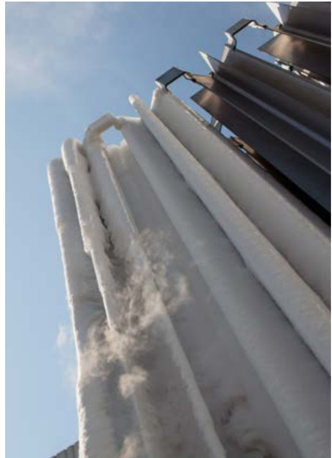
Bulk liquid nitrogen vapourisers
