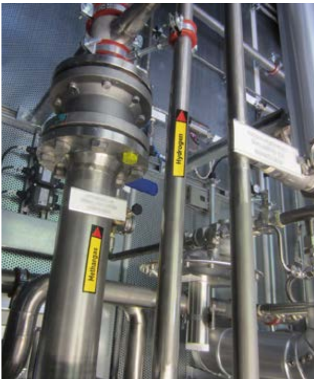
Hydrogen gas grid admixing. Copyright TÜV SÜD.
