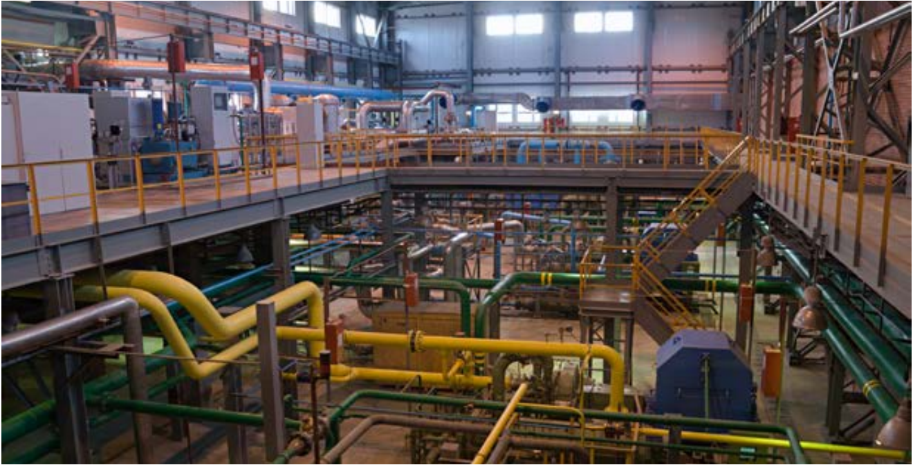
Motors, gas compressors and piping – an ASU machine room has many potential gas leak hazards
