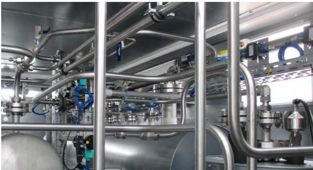
Hydrogen electrolyser installation. Copyright TÜV SÜD.
