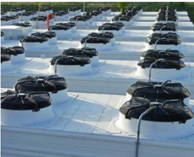
Ammonia refrigeration system evaporators
