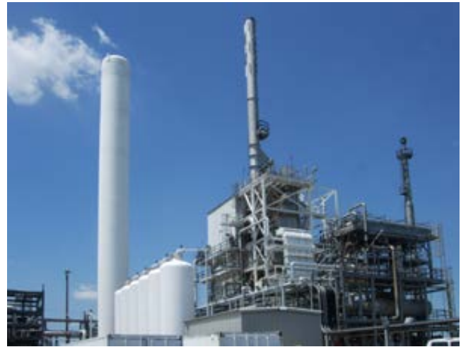
Steam Methane Reformer (SMR), Lima hydrogen cluster, Ohio – copyright Matheson Tri-Gas
