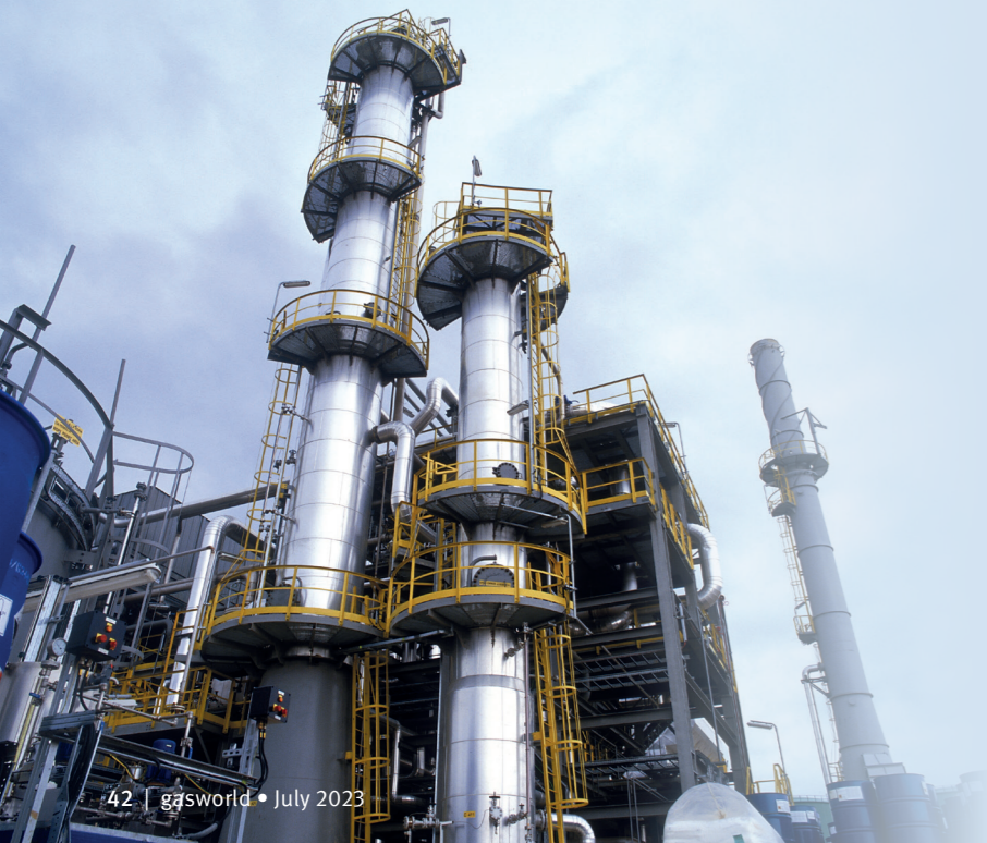
© APCI | CO 2 capture absorber and stripper towers.
