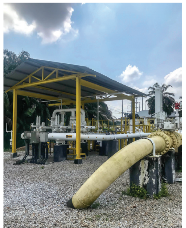
Gas pipeline flow and purity monitoring station
