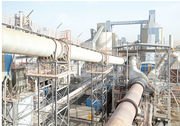
Copyright ABB, Cement making kiln
