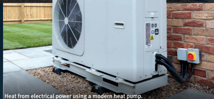
Heat from electrical power using a modern heat pump.
