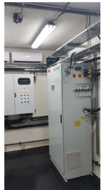
Copyright ABB - ACF5000 FTIR CEMS installation
