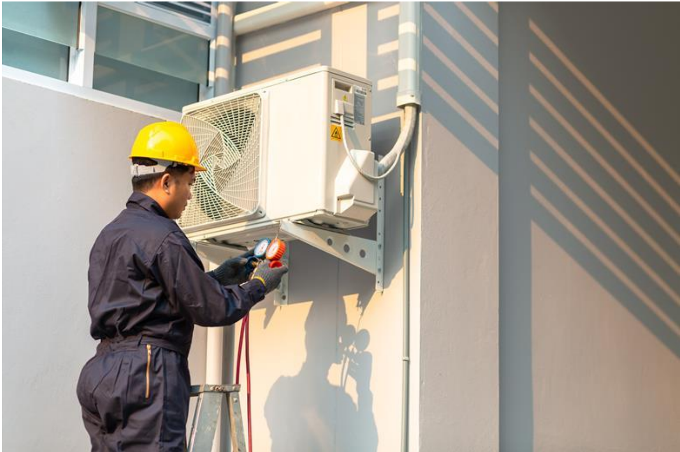
HVAC refrigeration F-Gas system maintenance
