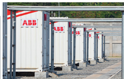
Above: ABB Limay battery installation includes the provision of battery enclosures, EcoFlex eHouses, UniGear ZS1 medium-voltage switchgear, and integrated skid units with transformers and inverters
