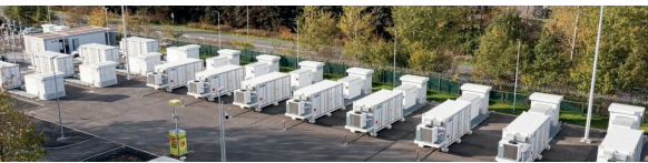
Above: RWE mega battery installation
