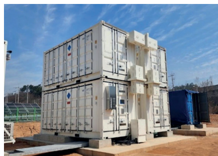
Above: NGK NAS battery installation at Kepco's Naju demo site
