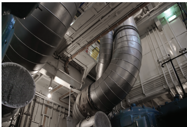
Ship's engine exhaust system
