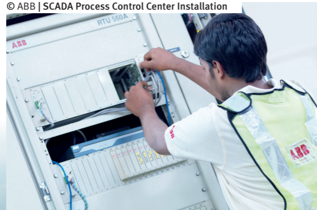
© ABB | SCADA Process Control Center Installation
