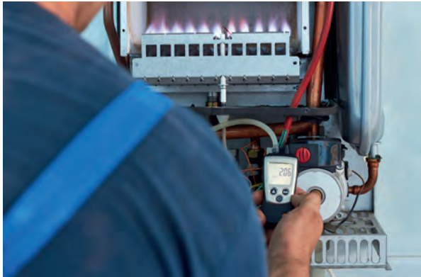
Flue gas testing on a boiler
