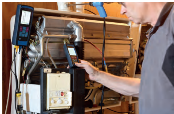
Maintenance and gas testing on an industrial boiler
