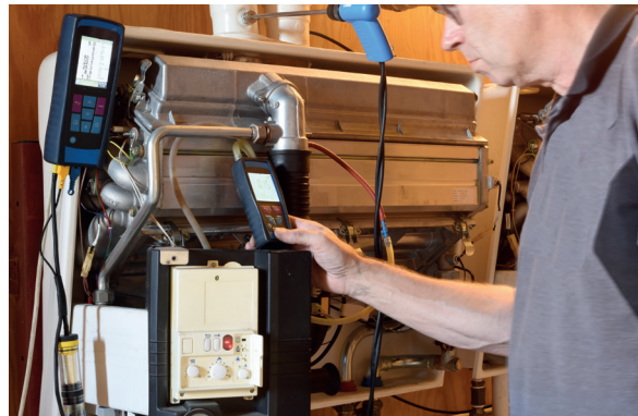
Maintenance and gas testing on an industrial boiler
