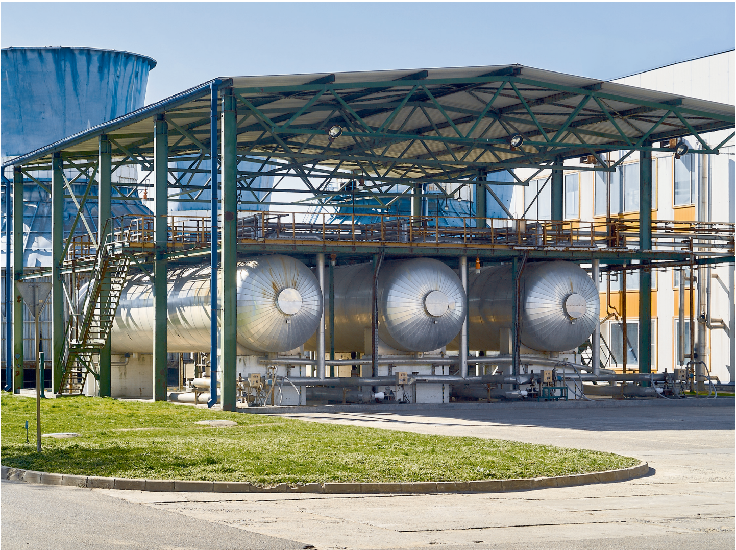
Cryogenic liquid CO 2 storage tanks
